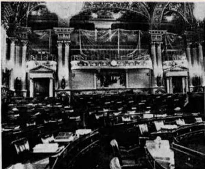
INSTALLING BULLET-PROOF GLASS —Workmen have installed plastic in the visitors gallery in the State House of Representatives in Harrisburg to control the dust as they prepare to install bullet-proof glass in front of the gallery between the visitors and the State Legislators. The work is expected to be completed by the end of August. (AP Wirephoto)
